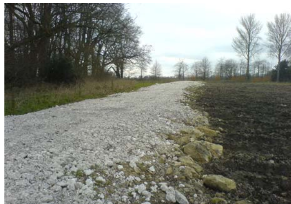
Fig 4: Investing effort in preparing a raised base will improve drainage. Some 'sinking' should be anticipated and an 'over-camber' is rarely the main concern.
