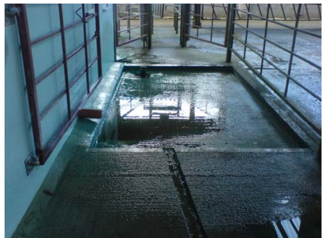
Fig 7: A double width bath with bung, over-flow, and parlour washing divert
